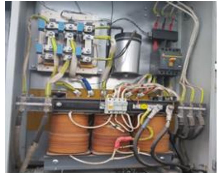
Charging station of the trolleybuses
